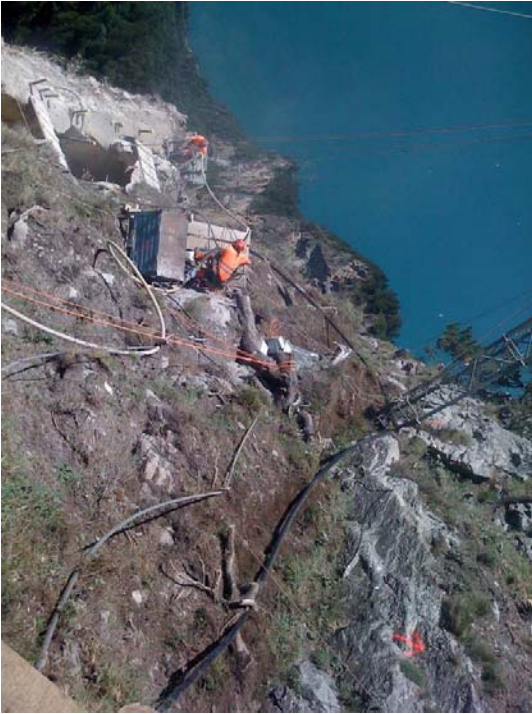
Rock and ground monitoring Switzerland
